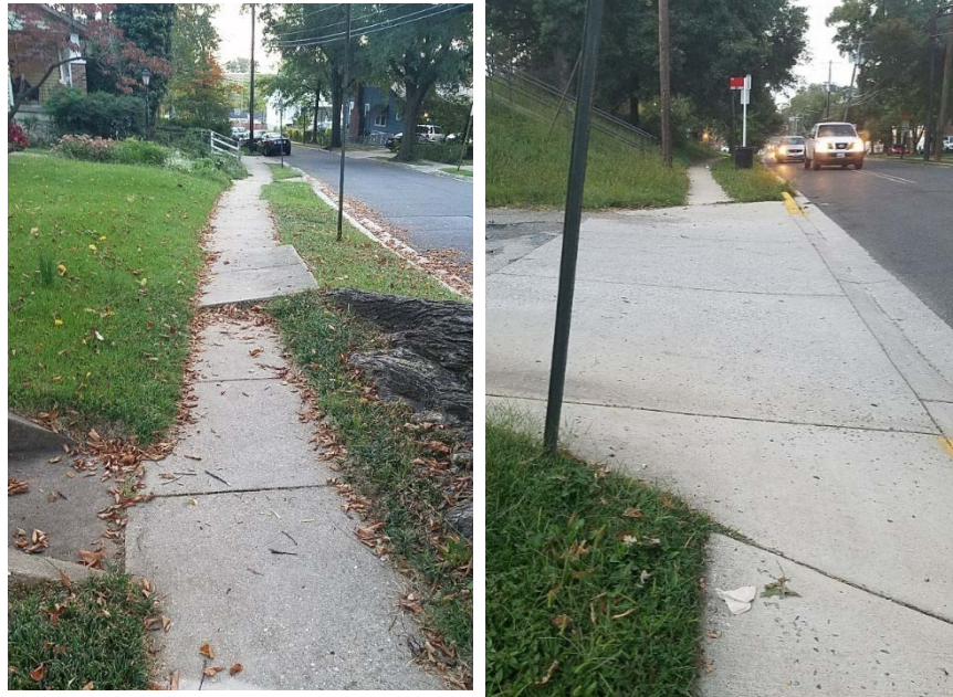
Figure 18: Uneven Sidewalk (left) and sloping driveways create access management issues on sidewalks (right)
