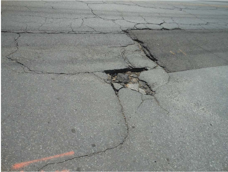
Figure 23 - Pothole in the bicycle lane/Trail, southbound at Fox Street.
