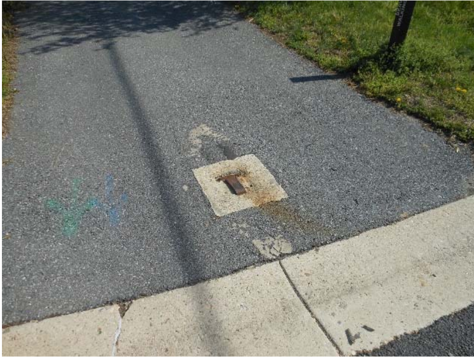
Figure 35 – Missing bollard at Quebec Street; one of several missing bollards in the Berwyn area.
