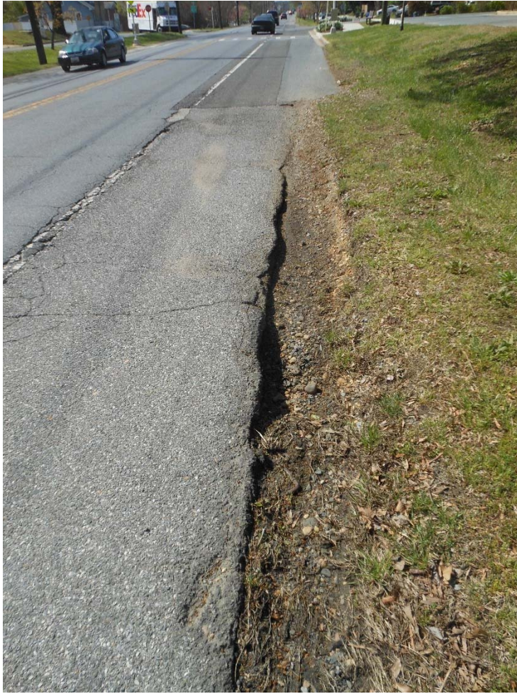
Figure 24 - Roadway erosion, approximately 7 to 8 inches deep, of the southbound bicycle lane/Trail, located 100 feet north of Fox Street.
