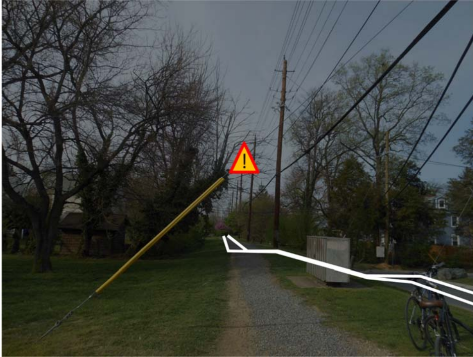
Figure 30 - Northbound view from the private parking lot just north of Berwyn Road. The low powerline is hazardous, especially during the hours of darkness, for both northbound and southbound Trail users who cut through the private parking lot, instead of following the appropriate Trail path.
