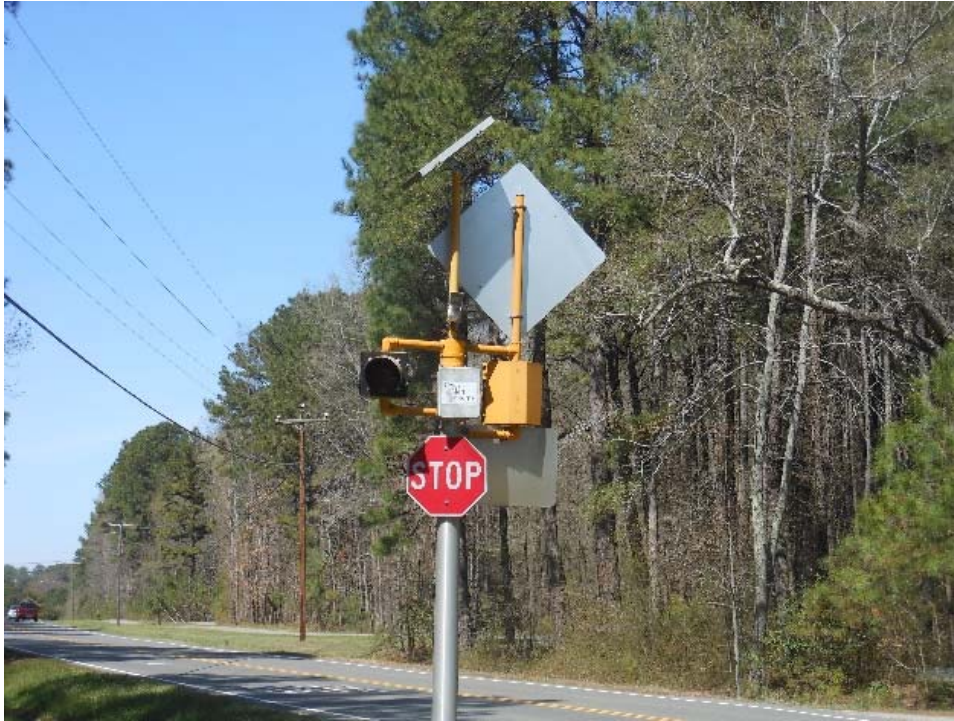
Figure 25 - Example of a traffic control device, used on another trail, at a dangerous crossing.
