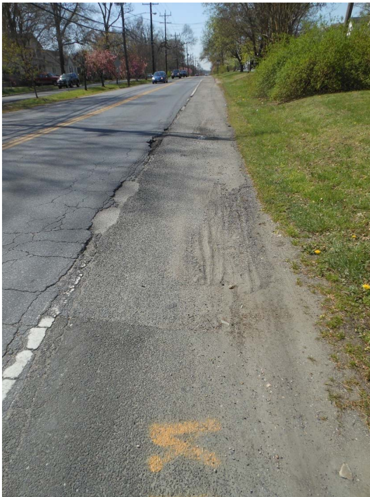
Figure 21 - View of sand and debris build-up in the bicycle lane/Trail near Hollywood Street.
