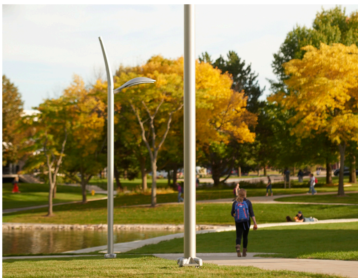
Site Lighting & Security Cameras
